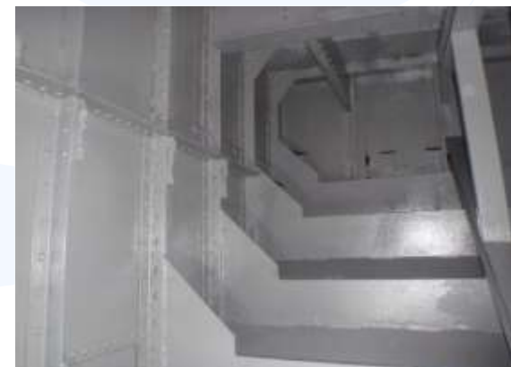
Photographs: • No. 1 Condition of the barge after jet washing • Nos. 2 and 3 The ballast tanks condition after stripe and full coat of RS 500P
