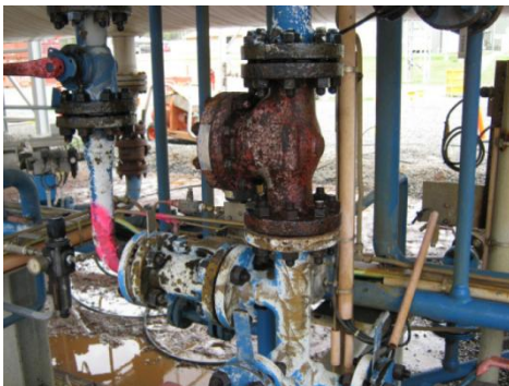
Before – Ammonia Bullet Pipelines
