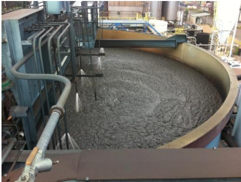
Plant in operation
