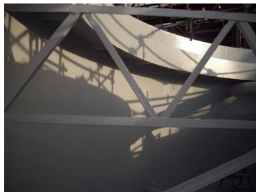
Launder and steelwork
