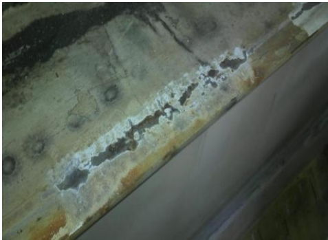
Mechanical damage with heavy pitting
