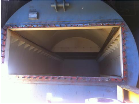
32 year old heat exchange vessel
