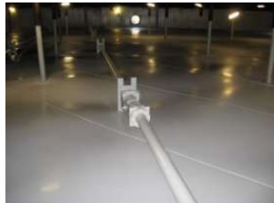
Epo-chem™ RA 500M Crude Oil Tank
