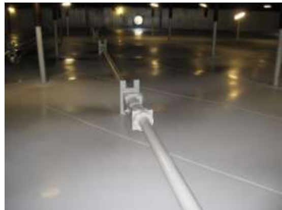
Epo-chem™ RA 500M Crude Oil Tank
