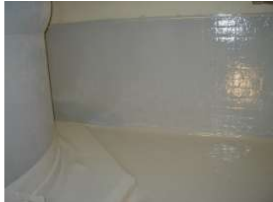
Epo-chem™ RF 500 Bund Lining
