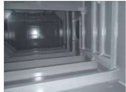
Potable Water Tank
