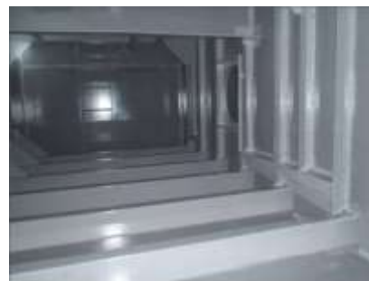
Potable Water Tank
