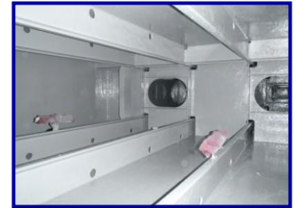
Completed application consisting of one stripe coat (RS 500P), one primer coat (RS 500P) and one topcoat (RA 500M)
