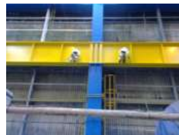
Easi-gloss™ RX 500GS Turbine Hall Structure
