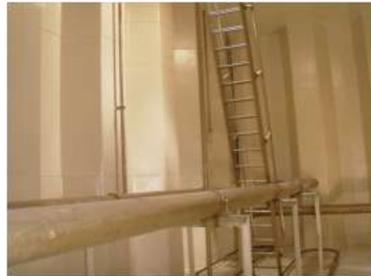
Completed project - 2 x 500µ DFT Chem-TECT™ RB 364 applied to a Sa 2½ grit blasted surface
