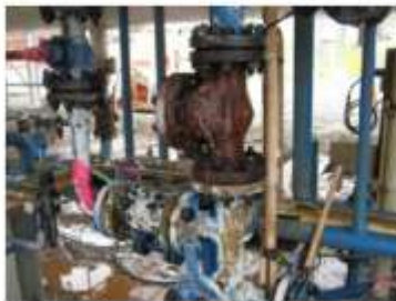
Before – Ammonia Bullet Pipelines
