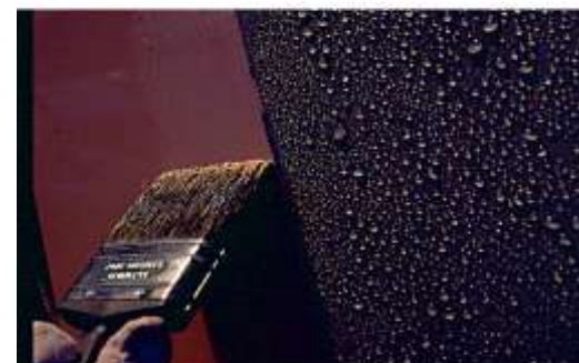
RS 500P on a sweating and damp surface
